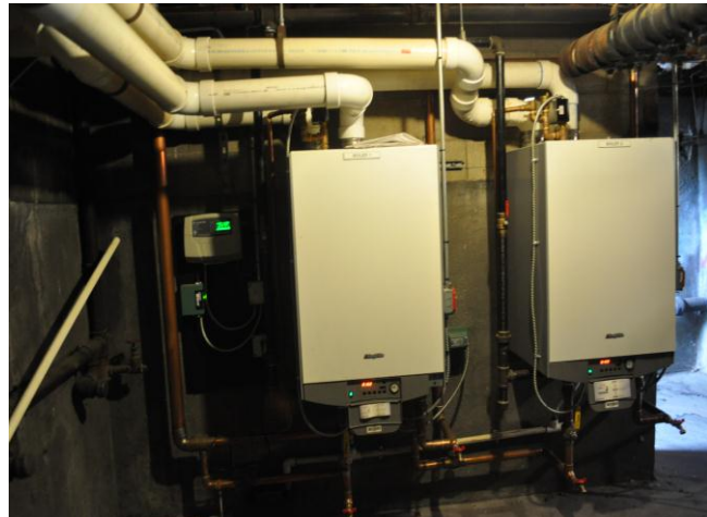
New Gas Boilers
