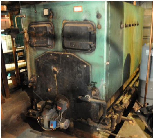
Old Oil Fired Boiler
